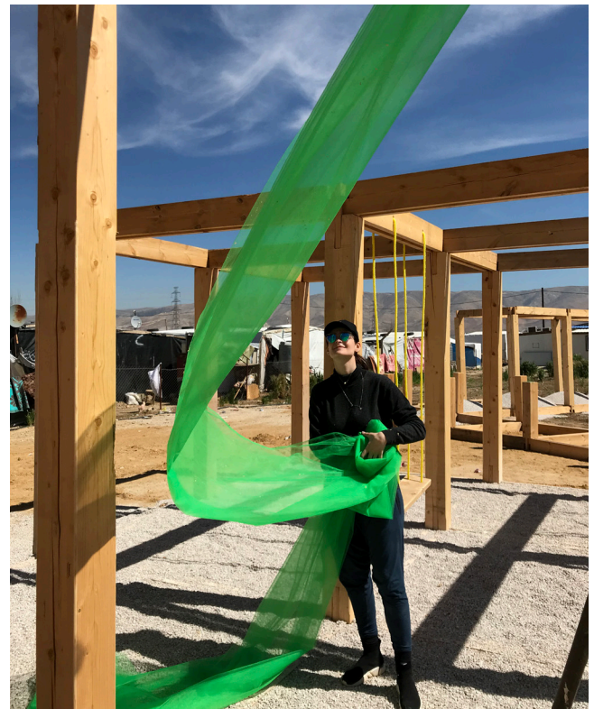
Figure 13: Project Architects actively participated in the construction effort, engaging with camp residents and children.
